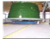
Step 3: In this photo, the support jacks are deployed to support the mold during gel coat spraying. Source: Matrasur
