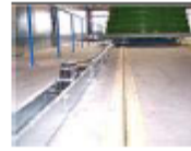
Step 1: The parallel tracks and moving conveyor used to move the pool molds around the carousel, during facility commissioning. Source: Matrasur
